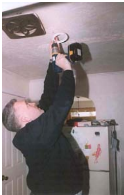
Always have a working Smoke Alarm
